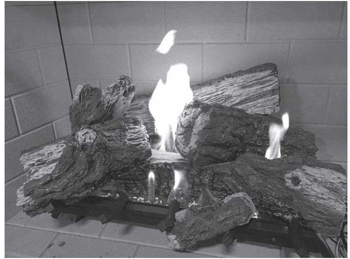
Figure 6.13 - Correct Appearance of Rear Flames
