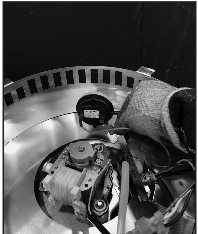
Figure 5.3 Remove Wires from Pressure Switch
