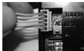
Figure 20 - Connecting end of Touch Pad Cable
