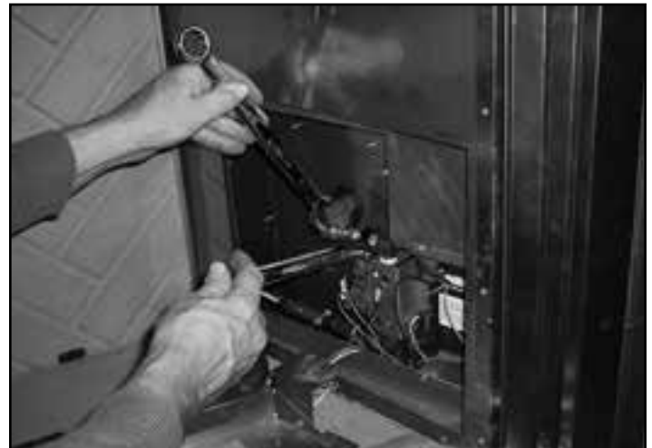
Figure 12.6 Turn off Gas Valve
