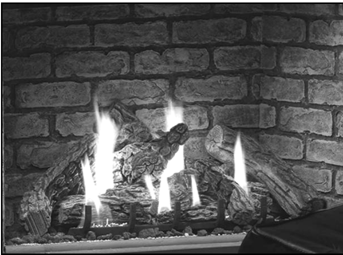
Flame should appear similar to the above picture.
